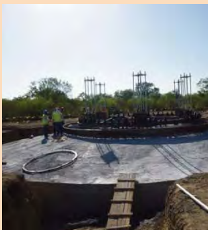
Ventika Wind Farm
